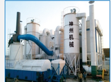
Drying-Dry Separation System
